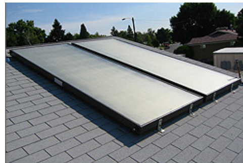
Figure 16: Solar hot water collectors
