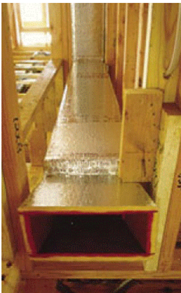
Figure 7: Duct in floor
